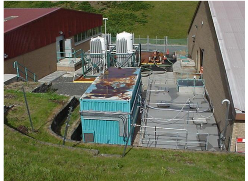
Ozone Plant at Glenfarg WTW
